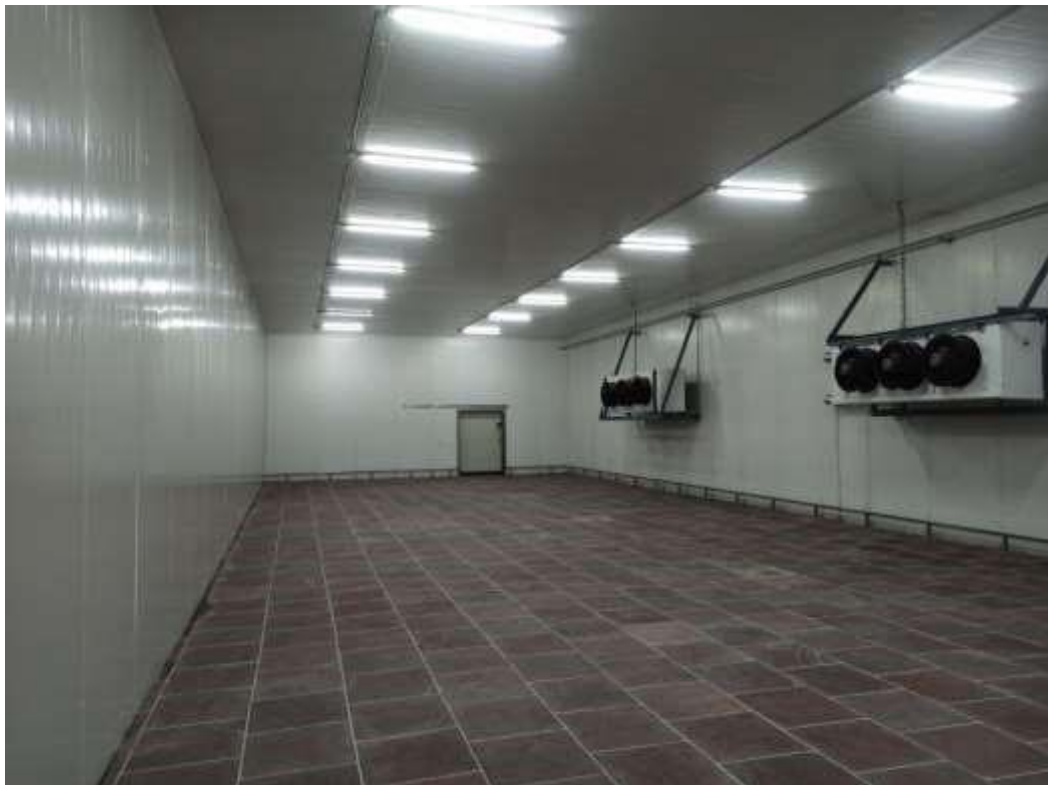
Fig.14: Cold storage room
