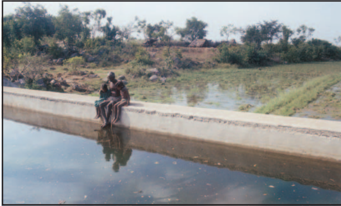
Checkdam on a drainage line
